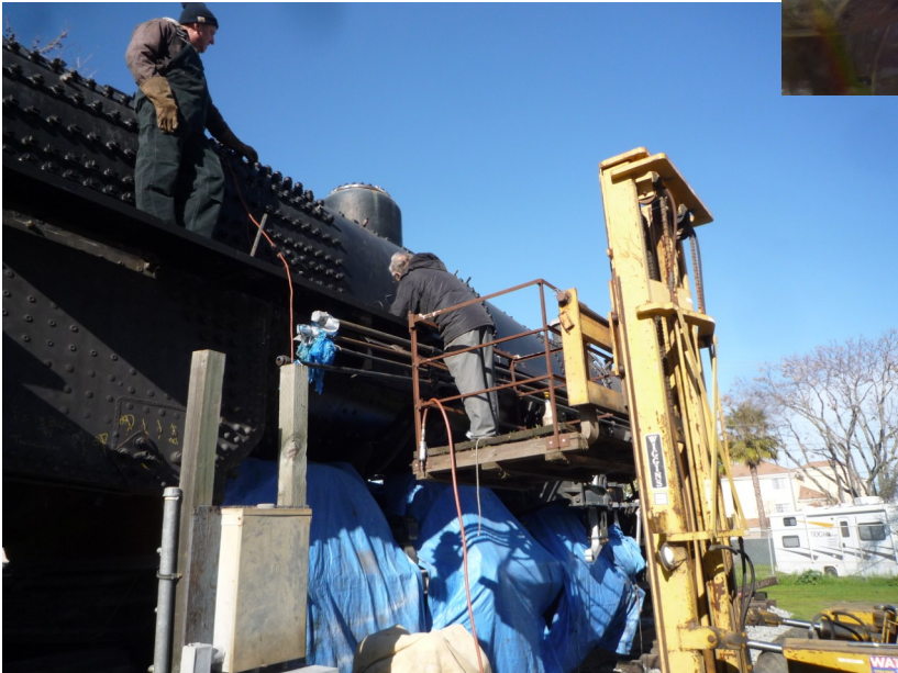
← the balance spring mechanism for the reverse cross shaft has been re-installed, as have the hangers from the cross shaft arms to the radius rods,
